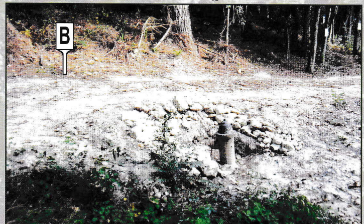
FIRE PLUG EXCAVATED: surprising amount of silt had accumulated across time to the extent that all but the top of the fire plug was covered. Also, the huge shed was close to the plug.
